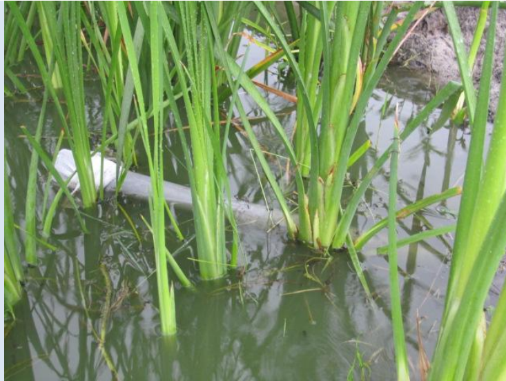
Outlet pipe to allow excess water to drain from the pond
